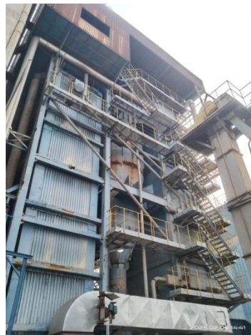
Gambar 3: Boiler CFB Kapasitas 50 ton/jam
