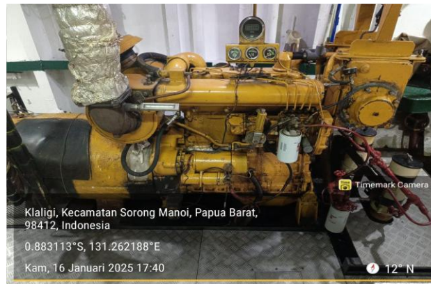
Gambar 4: Motor bantu KM Binama No.7
