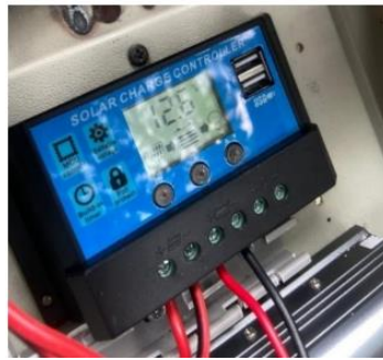
Gambar 3. Solar Charge Controller tipe PWM
