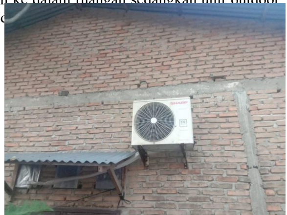
Gambar 5. Gambar Unit Outdoor Air Conditioner
